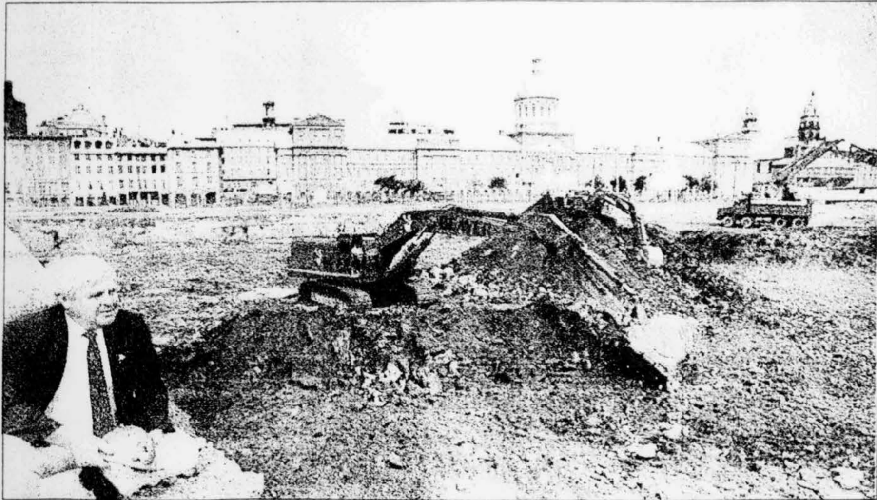
Al Wiebe, general manager of Beaver Construction, supervises excavation of an artificial lake being built near Bonsecours Market to celebrate Montreal's 350th birthday.
