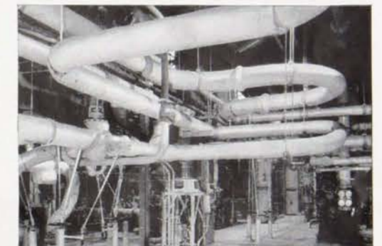
S & L design, manufacture and erect steel pipe-work installations for all types of industrial power plants.
