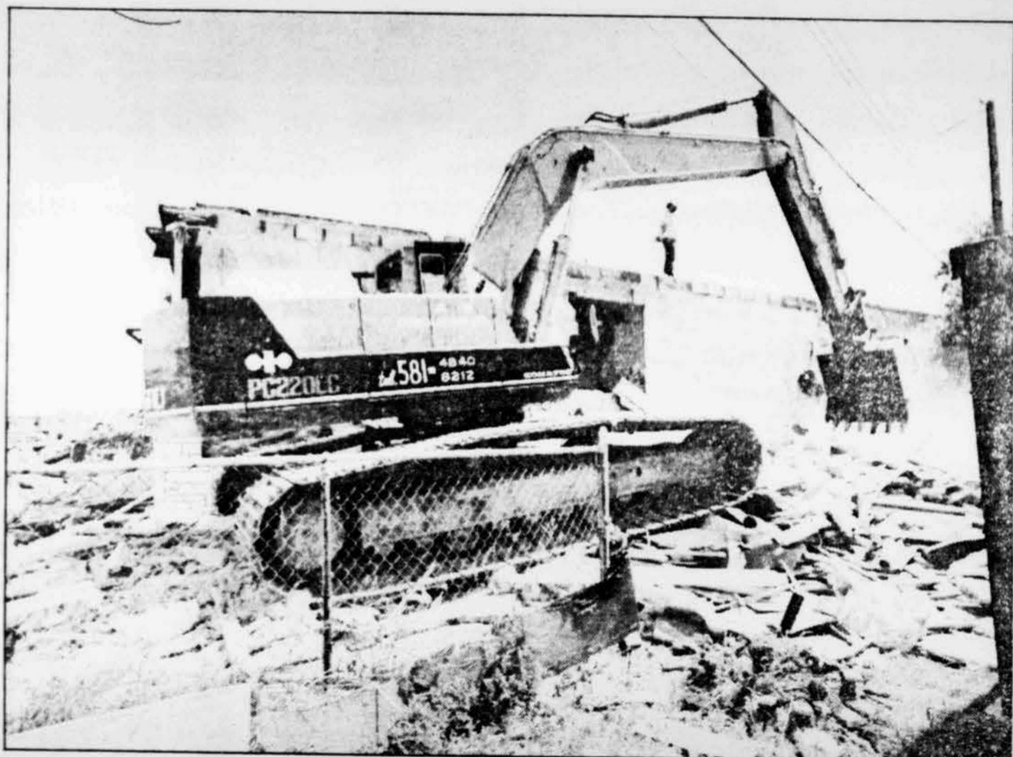
Eight LaSalle duplexes are being demolished to make way for toxic waste cleanup in former dump. Gazette, Len Sidaway
