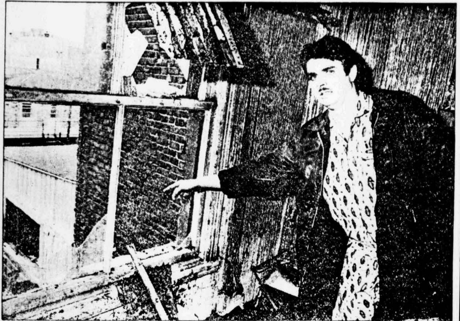
Guy Deschambault points to window he escaped through as flames engulfed apartment at 1693 Amherst St.
