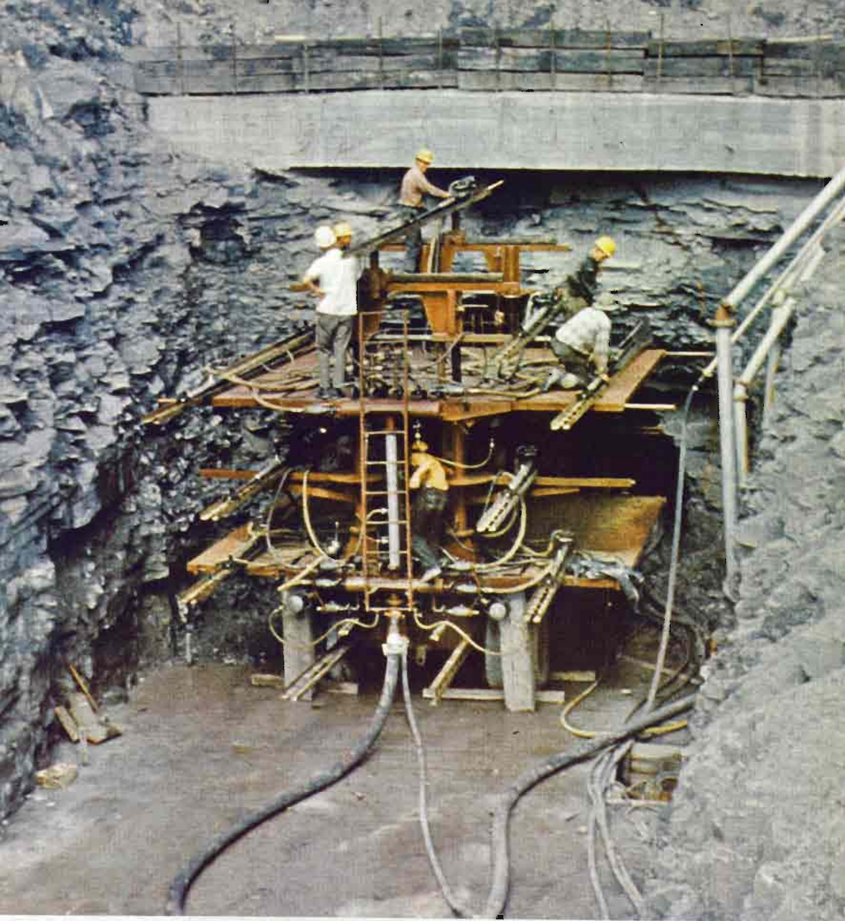
Foreuse type "Jumbo" à l'oeuvre ● Machines aid man in tunnelling work ● Perforadora tipo "Jumbo" en pleno trabajo ● Perforatrici "Jumbo" intaccano la roccia ● Bohrmaschine "Jumbo" am Werk.
